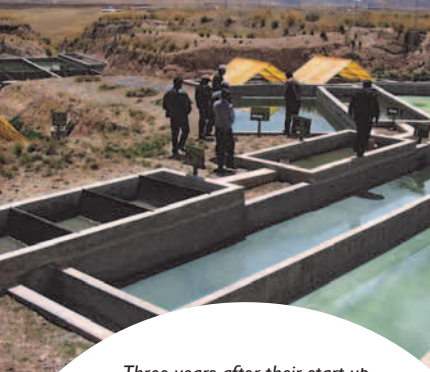
Three years after their start-up, the treatment plants of Choquehuenca and San José have their imitators. (Care)
